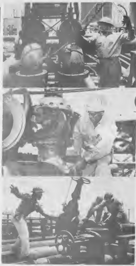
AN ELBOW is removed, top photo, by T. Geerman, helper A, and the stub, center, is inspected for leakage under pressure, W. Bailey, tradesman A, directly a valve as it is lowered onto a stub.
